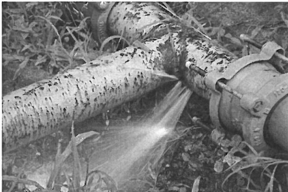
Example of maintenance issue at a water treatment facility. According to local sources, this leak has been on-going for several weeks unrepaired. It is estimated that this leak generates a water loss of about 1 2,800 Imperial gallon per day or 1 MIG per year
